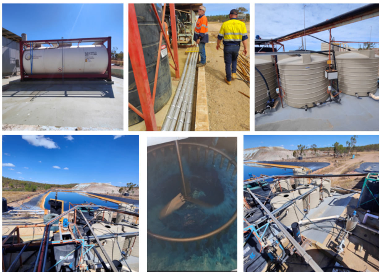
Figure 1. Tartana Solvent Extraction – Crystallisation Plant. Clockwise – New acid tanks with delivered acid, Inspection of pipework, New tanks for copper stripping, View of plant tanks and pipework, Copper sulphate crystals in crystalliser, Plant, PLS pond and heaps for leaching in distance.
