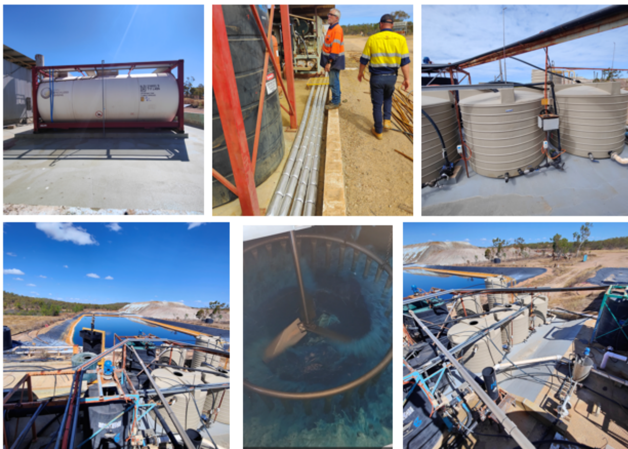
Figure 3. Tartana Solvent Extraction – Crystallisation Plant. Clockwise – New acid tanks with delivered acid, Inspection of pipework, New tanks for copper stripping, View of plant tanks and pipework, Copper sulphate crystals in crystalliser, Plant, PLS pond and heaps for leaching in distance.
