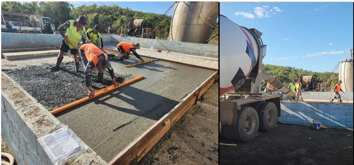
Figure 7: Civil works associated with the Sulphur acid tanks bund and pad, 27 May 2022.
